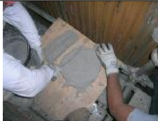
Figure 7: 15R is laid out on a mortar board prior to being installed
