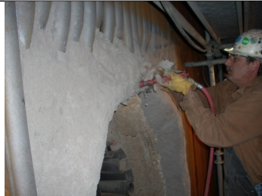
Figure 9: Thermbond Formula 15R being rammed in burner throat bring it back to its proper profile
