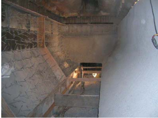
Figure 10: Wet bottom ash hopper with anchors in place and ready for gunning
