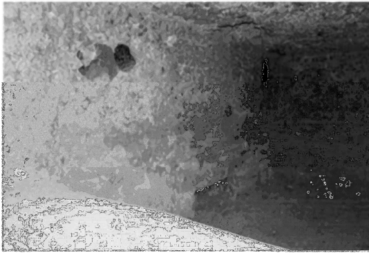
Figure 5. Same furnace wall shown in Figure 4 one year after reline with liquid phosphate-bonded refractory.
