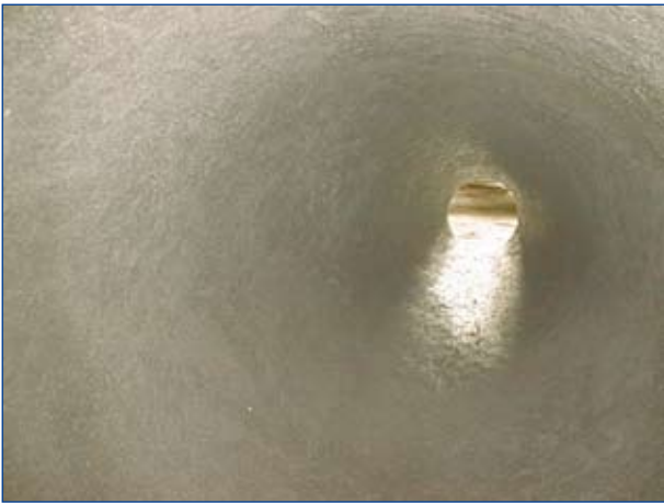
Figure 6. FCCU cold wall reactor riser.
