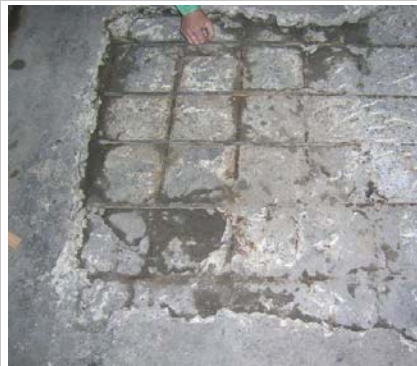
Damaged floor with rebar exposed.
